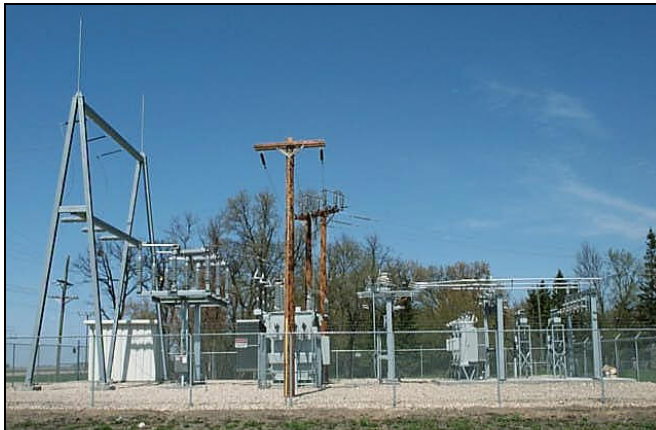
Fig. 1. Real electrical substation
